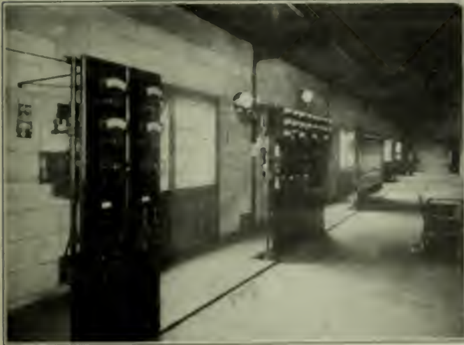
SWITCHBOARD GALLERY IN POWER HOUSE
